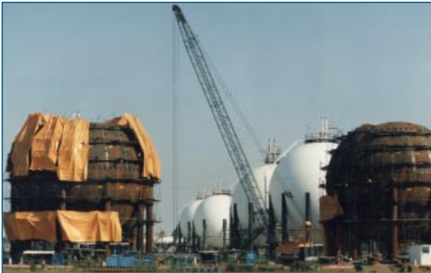
Liquid natural gas tanks under construction constitute a hazardous location where zone-classified products could be used.
